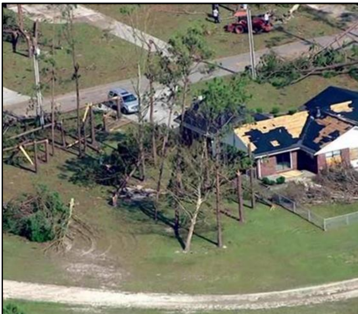
DAMAGED HOME IN WEWAHITACHKA
