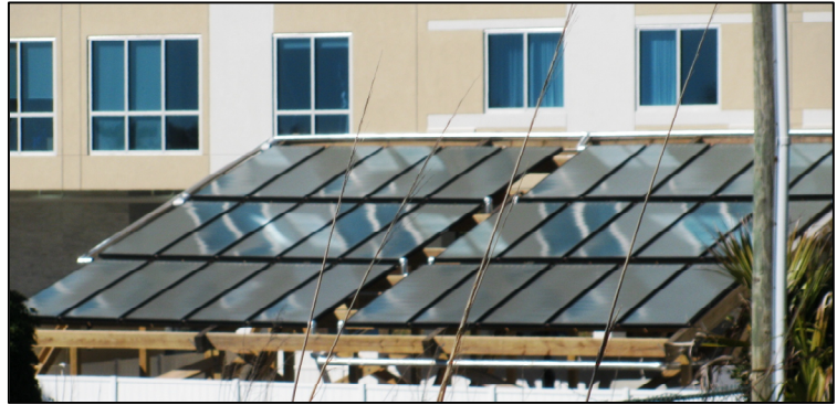
OKALOOSA ISLAND'S COURTYARD MARRIOTT SOLAR ARRAY (Located on the beach side of the building)
